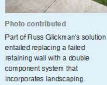
Photo contributed Russ Glickman re-graded the existing slope so that it never rises faster than one inch per foot. The ramp and deck flooring are constructed of Fiberon planks, which are durable and skid-free.
